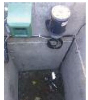
Flow and pressure meter
