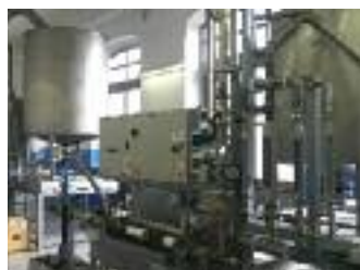
MM meter testing facility
